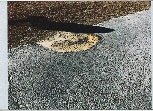
Photo 6. View of severe edge distress.
