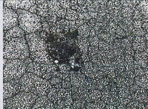
Photo 4. View of severe block cracking and raveling.
