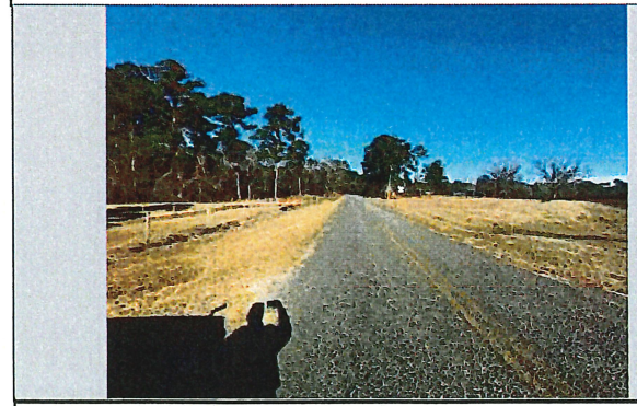
Photo 5. View of surface treatment with raveling.
