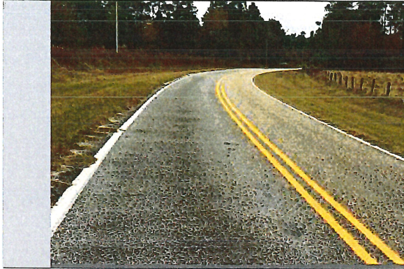
Photo 1. View of pavement damage on surface treatment.
