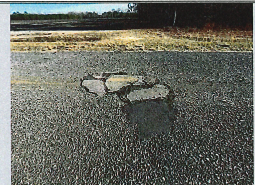
Photo 4. View of severe distress and pot holing.
