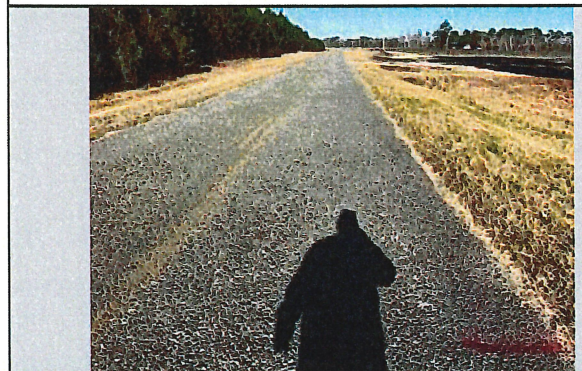
Photo 3. View of surface treatment w/ raveling.
