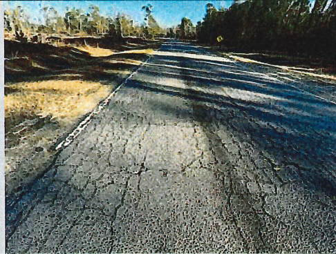
Photo 4. View of severe pavement block and load cracking.
