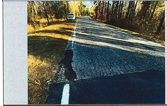
Photo 5. View of pavement load cracking w/ potholes.
