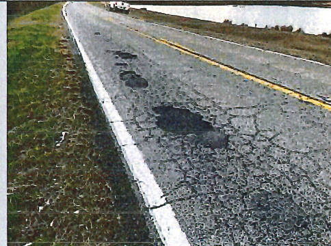
Photo 6. Failing Pavement Popping Out
