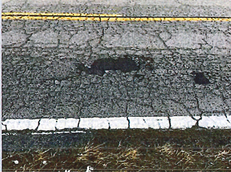
Photo 5. View of sever block cracking with failure
