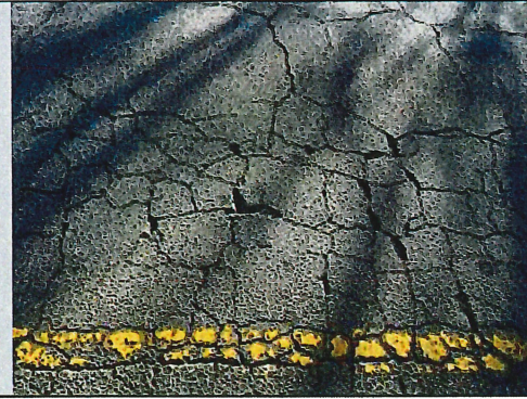
Photo 6. Severe Pavement load cracking with Popping Out
