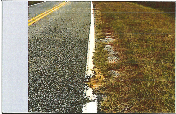
Photo 5. View of surface treatment with edge distress.
