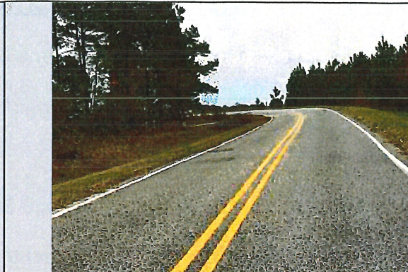
Photo 2. View of surface treatment pavement raveling.
