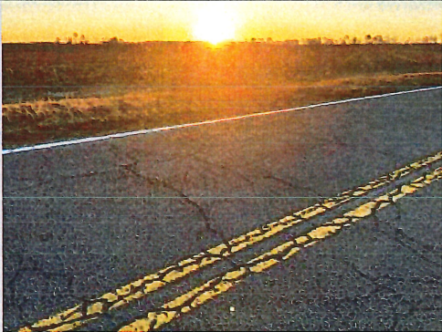
Photo 3. View of Block Cracking along Roadway
