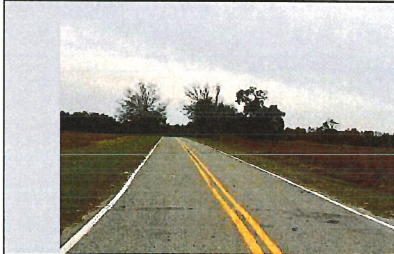
Photo 3. View of surface treatment raveling.
