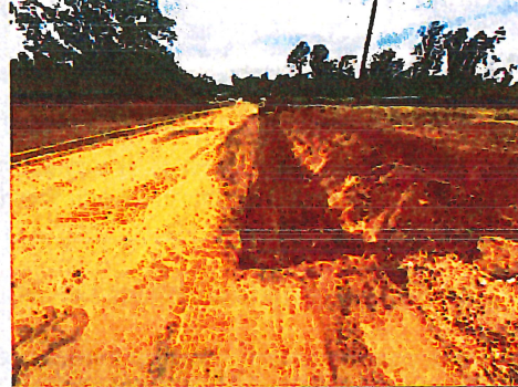
Photo 4. West Bound Lane Soft Spot Under Cut
