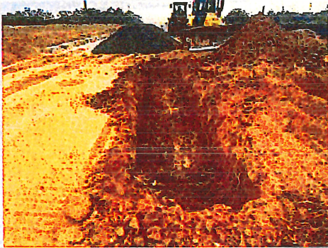
Photo 3. East Bound Lane Soft Spot was Under Cut
